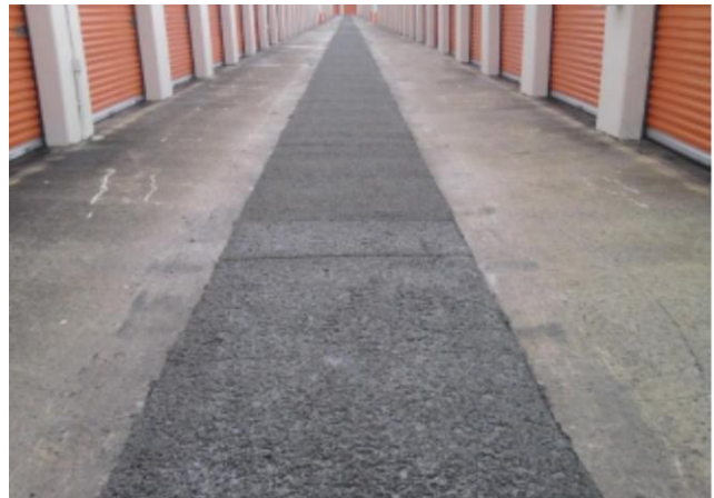
Aisle 2 - Photo taken October 21, 2011, two minutes after rain storm, with pervious pavement installation.
