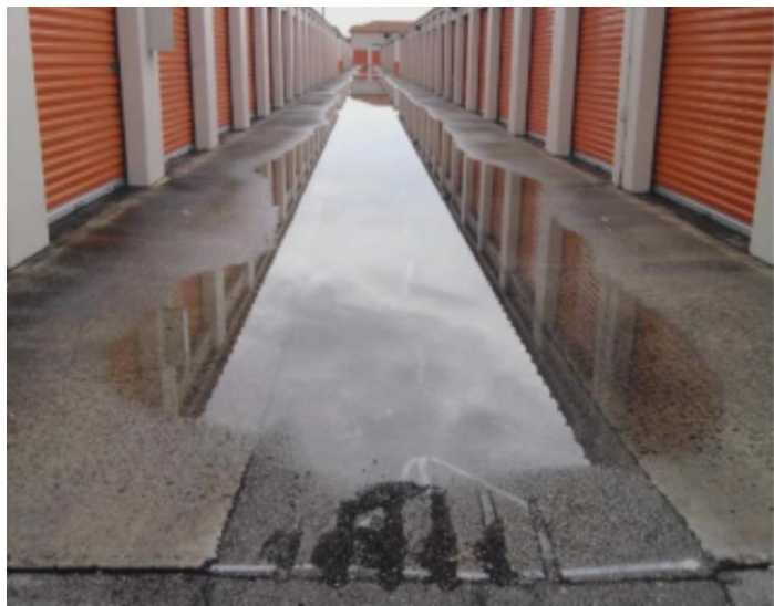
Aisle 1 - Photo taken October 21, 2011, two minutes after rain storm, without pervious pavement installation.
